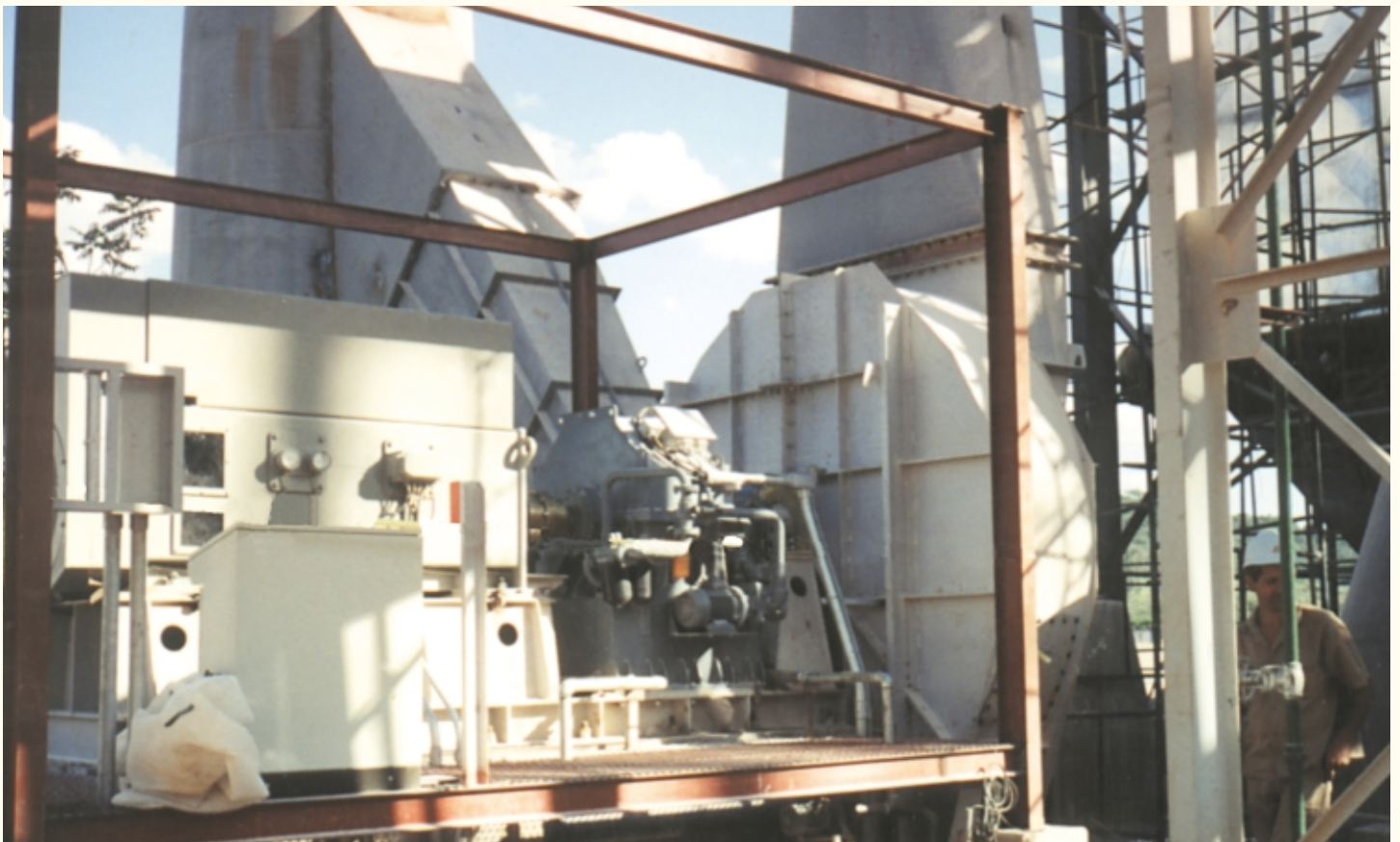
34 KSL, variable speed drive 700 kW - 1200 rpm, fan (Brasil)
